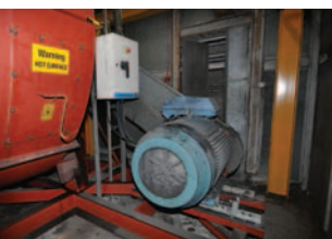
Drives can usually be accommodated in the plant room, in this case with a 180kW exhaust fan motor
